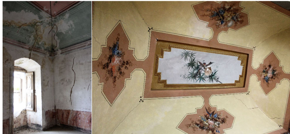
Figure 2. Examples of the crack pattern: corner walls (left) and vault (right).
