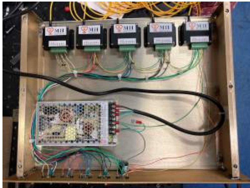
Figure 6.16. Photograph of the fully tested PoF transmitter module showing five 971 nm lasers.
