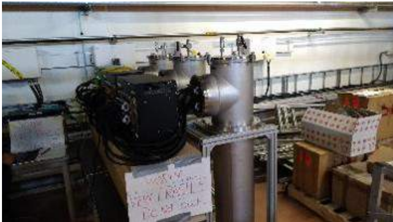
Figure 4.27. TDE integration test at EHN1 in summer 2021.
