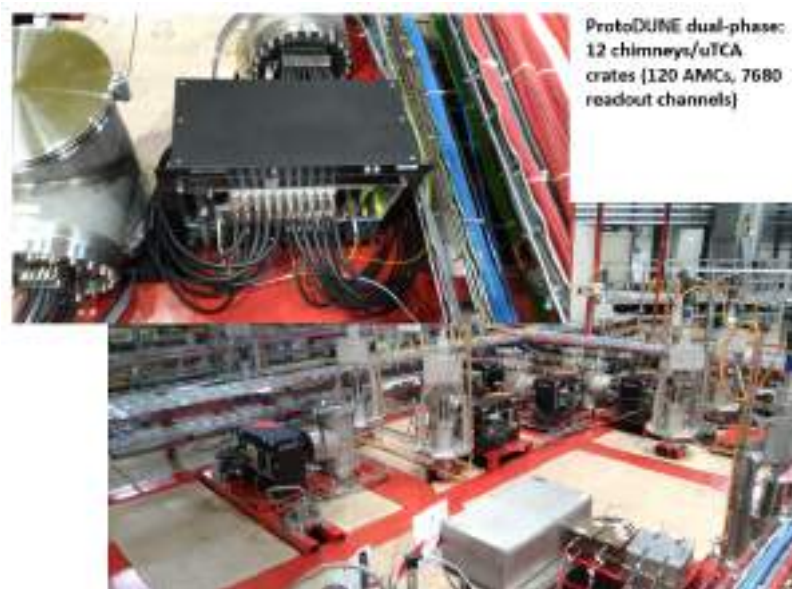
Figure 4.23. Charge readout system on the cryostat roof.
