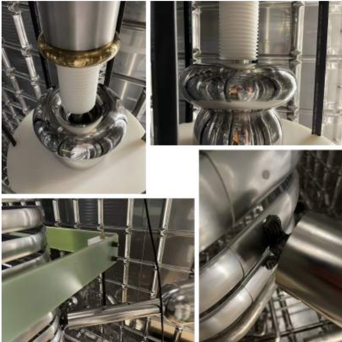
Figure 5.4. Components of the full scale HV long-term stability test in the NP02 cryostat. Top: two views of the doughnut and the sphere of the extender head with the HVFT tip connected. The gold colored ring in the top left photo is the sleeve to confine the gas bubbles produced by the heat input from the HVFT and evacuate them to the gas phase close to the HVFT ground skin. Bottom left: the tip of the extender in front of the field cage. Bottom right: detail of the extender connection to the field cage.
