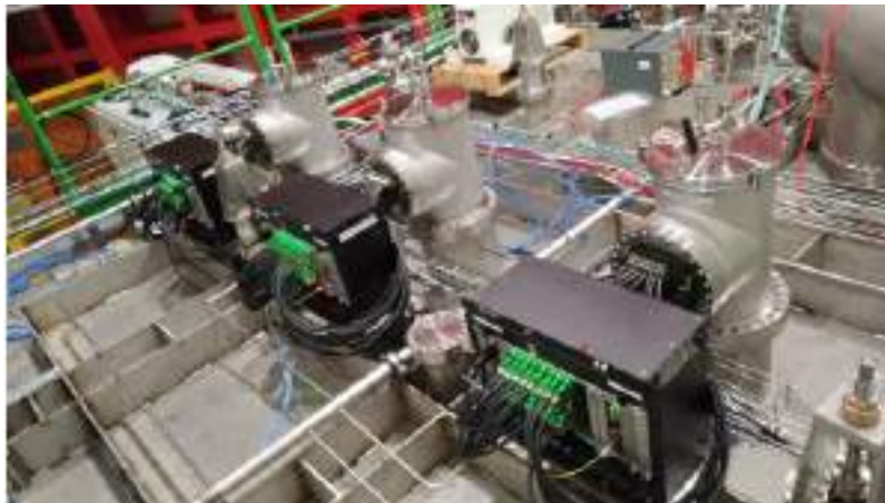
Figure 4.29. TDE installation on the cold box cryostat roof for the test of CRP-1.
