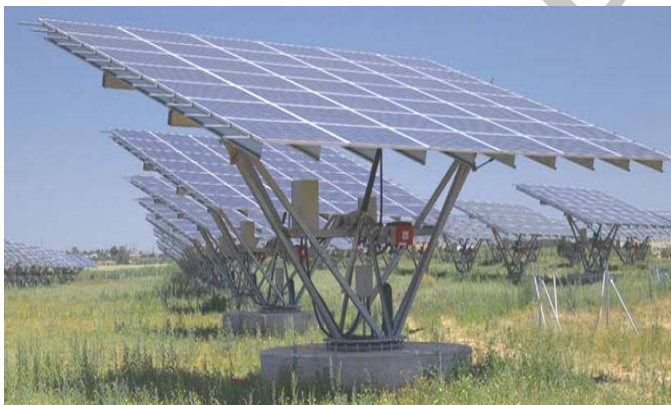
Figure 21. Photovoltaic plant with bi-axial solar trackers for final testing of the realized electronic equipment
