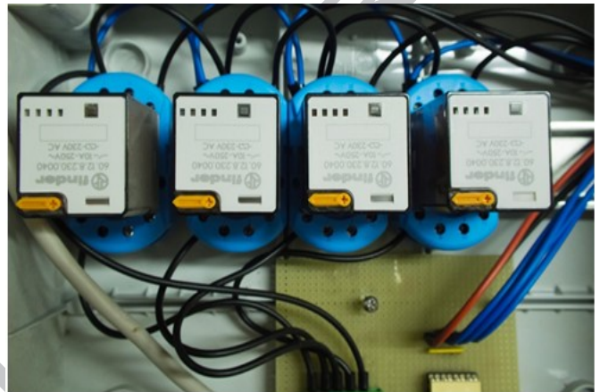
Figure 18. Zoom on the 4 actuation relays for motor control in the simulation block of the tracker motors.
